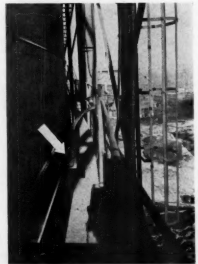
Fig. 3: Arrow indicates position of one of four steam jet syphons installed on the five million cubic foot holder.
